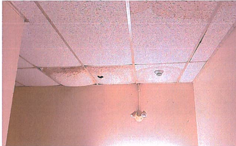
Photo 061 Signs of Moisture Damage
