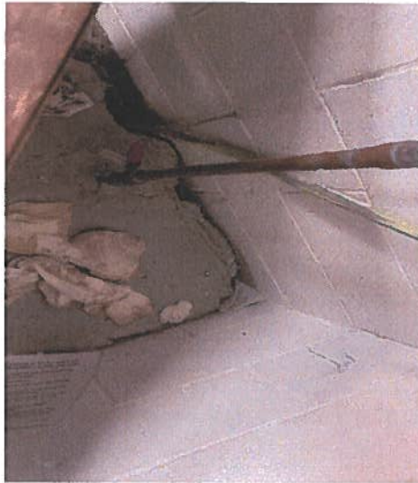
Photo 051 Slab-On-Grade to Wall Separation in Compressor Room
