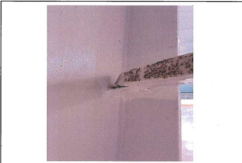
Photo 004 Rust on Frame Brace
