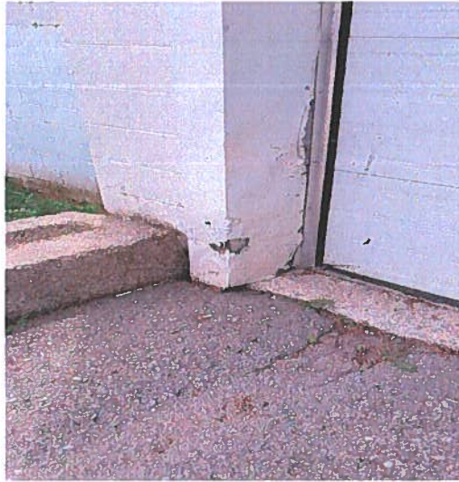
Photo 085 Damage to Garage Door Entrance
