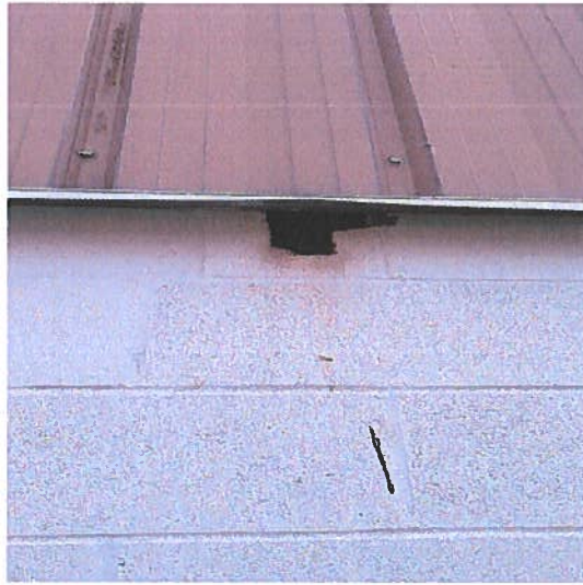
Photo 093 Hole in Masonry Block
