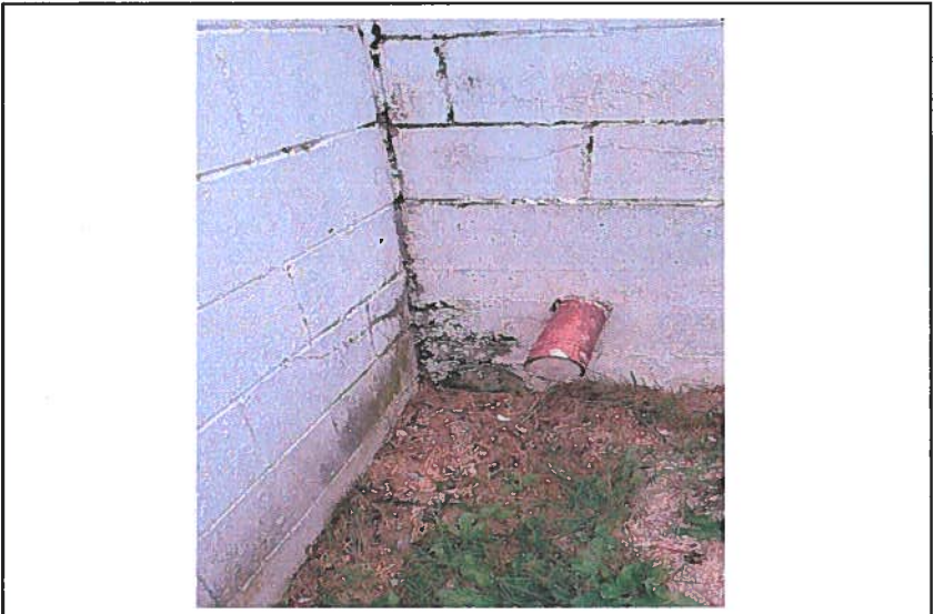
Photo 082 Honeycombing and Mould Growth
