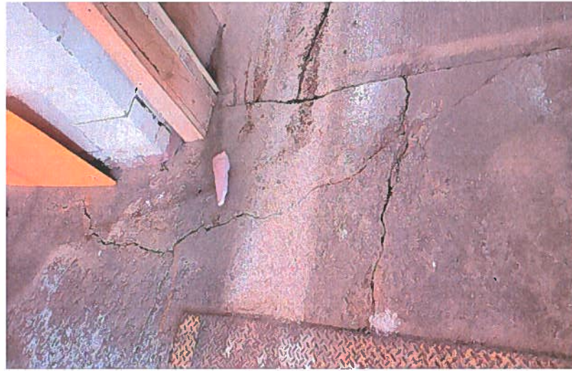
Photo 022 Extents of Resurfacing Room Cracking
