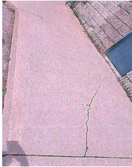
Photo 070 Damage to Sidewalk
