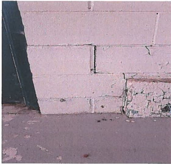
Photo 039 Step Cracking and Damage to West-Side Exit
