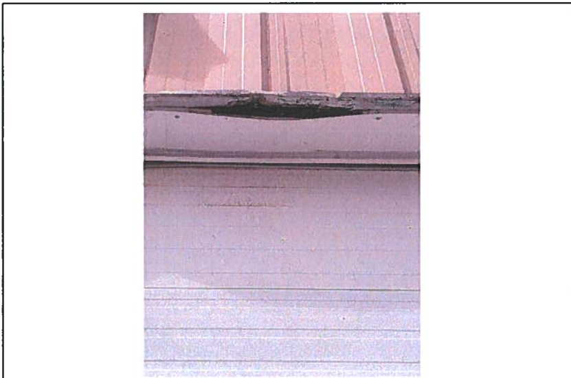
Photo 078 Close Up of Damage Garage Door
