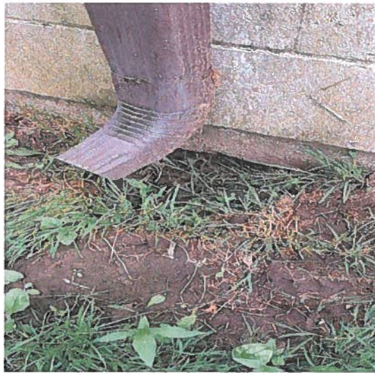
Photo 092 Localized Foundation Wall Damage
