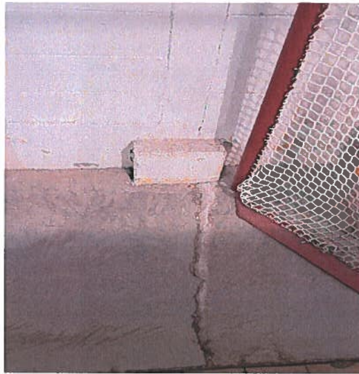
Photo 023 Cracking Under North-Side Column
