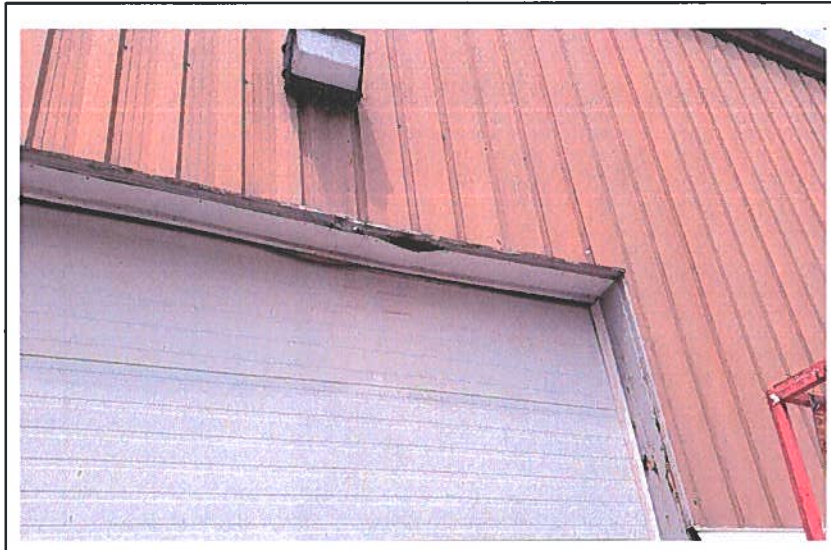
Photo 077 Damage to Garage Door Opening
