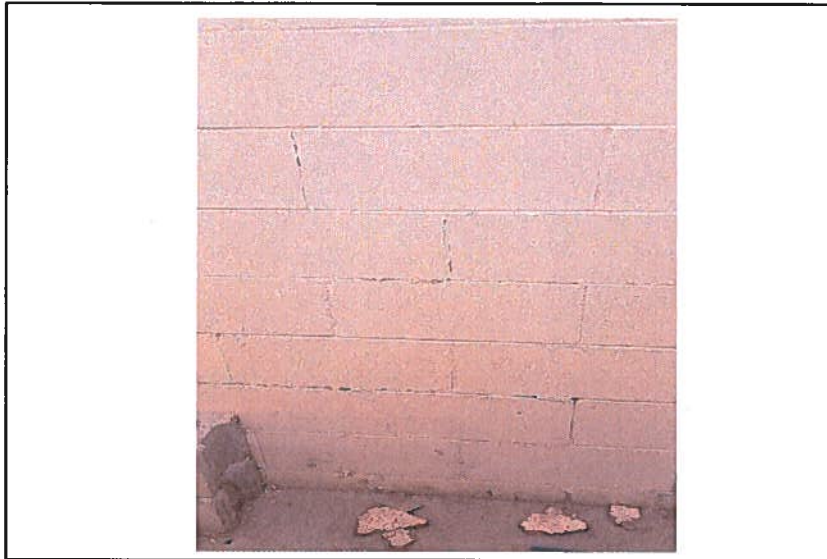
Photo 031 Minor Step Cracking in West-Side Stairwell
