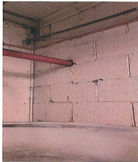
Photo 028 Multiple Step Cracks Behind Water Tank
