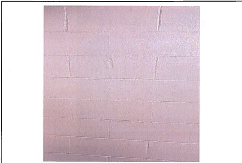
Photo 043 Localized Damage in Changeroom 3
