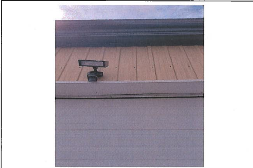
Photo 087 Damage to Garage Door Seal
