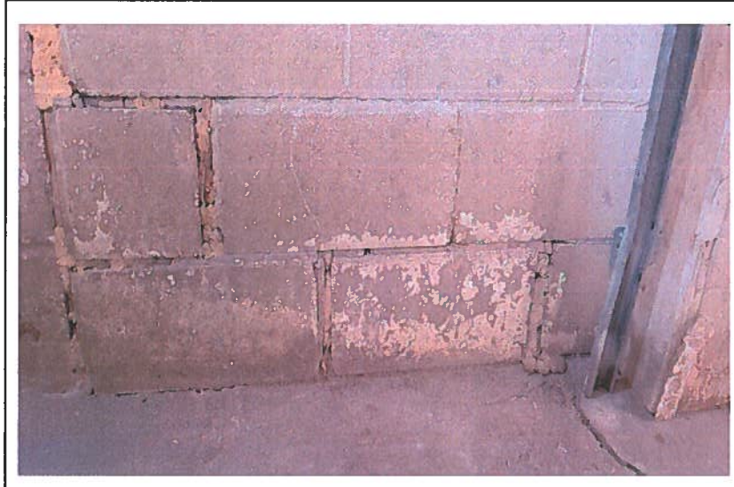
Photo 037 Existing Block Separation Repairs
