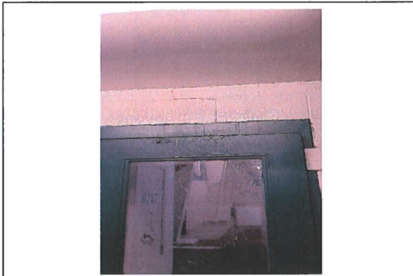
Photo 030 Step Cracking in Lobby
