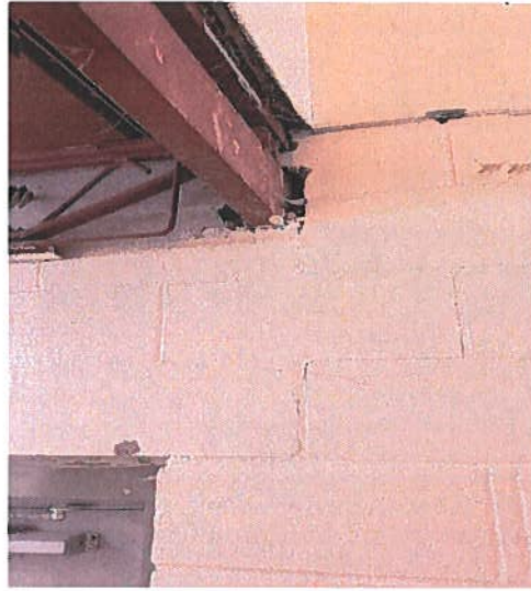
Photo 047 Localized Block Failure
