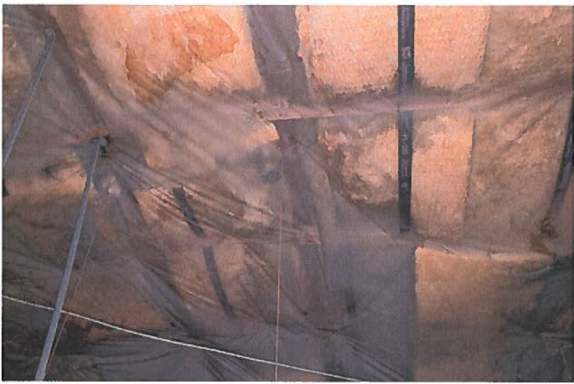
Photo 060 Moisture in Roofing System
