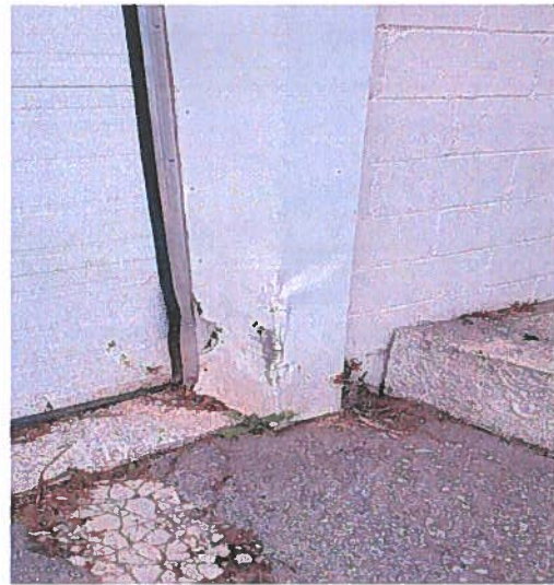
Photo 086 Damage to Garage Door Entrance
