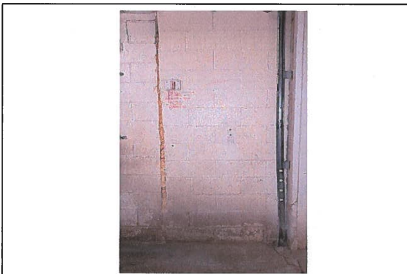
Photo 036 Differential Settlement in Ice-Resurfacing Room
