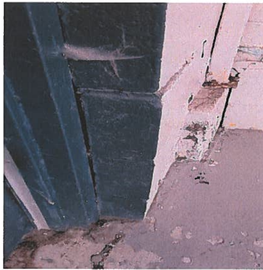
Photo 040 Wall Separation at West-Side Exit
