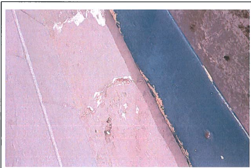
Photo 010 Paint Chipping and Crack on Bleachers
