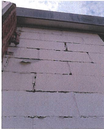
Photo 080 Step Cracking and Paint Peeling
