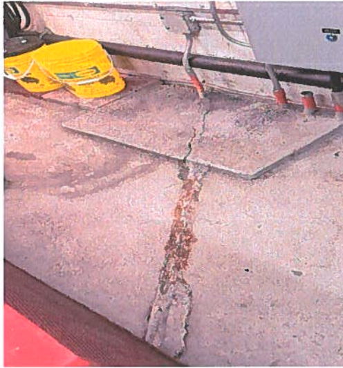
Photo 053 Concrete Damage at Electrical Equipment in Compressor Room
