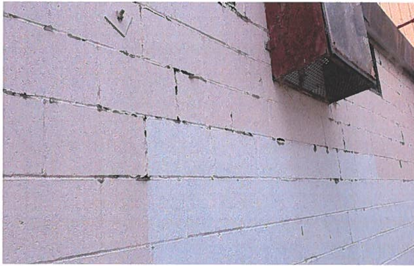
Photo 079 Step Cracking and Paint Peeling
