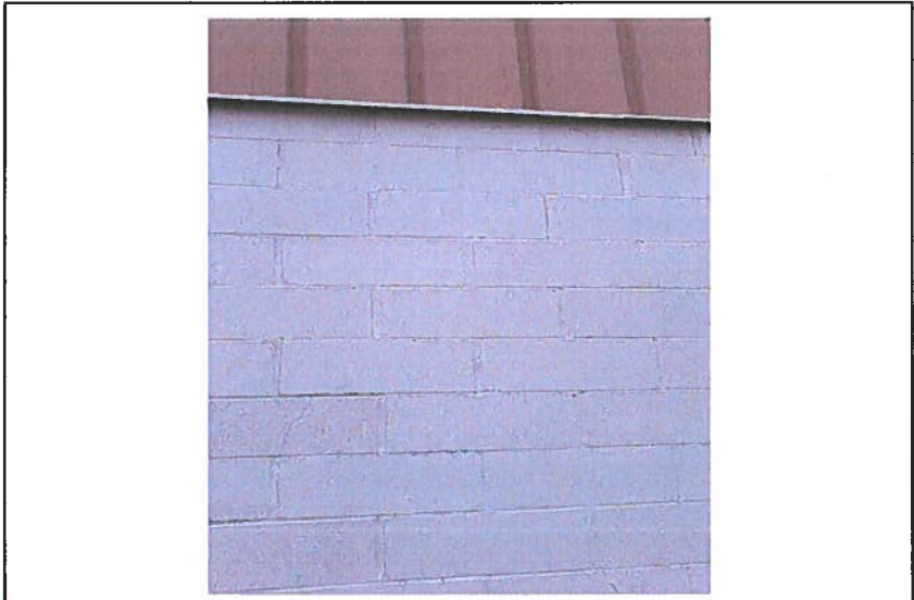
Photo 081 Step Cracking and Block Failure
