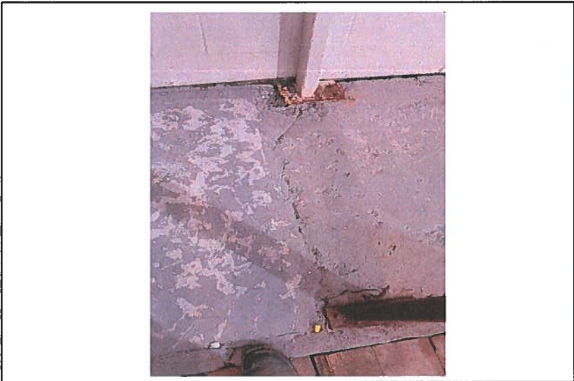
Photo 025 Crack Underneath Mechanical Equipment Stand
