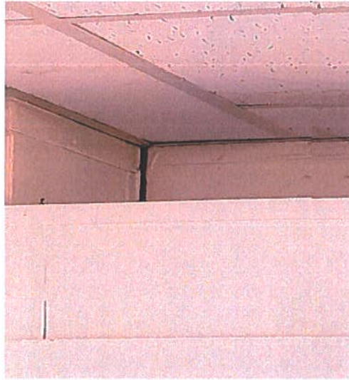
Photo 049 Wall Separation in Second-Floor Storage Room
