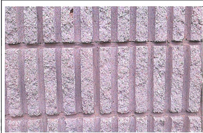
Photo 065 Architectural Block Mortar Cracks
