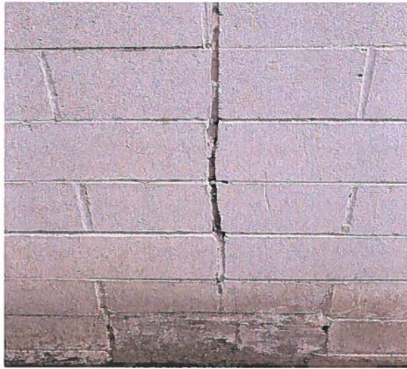
Photo 091 Damaged Wall Joint
