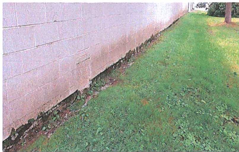
Photo 090 Mould Along West Side
