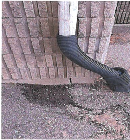
Photo 071 Gap in Foundation Wall
