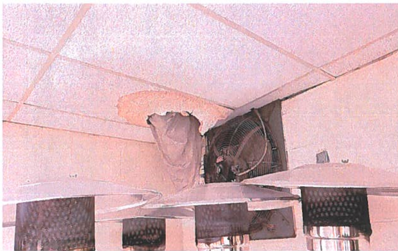
Photo 062 Signs of Moisture Damage
