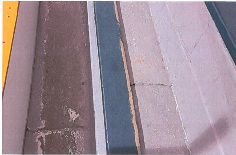
Photo 011 Bleacher Crack at Joint Location
