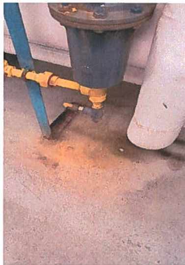
Photo 052 Concrete Staining in Compressor Room
