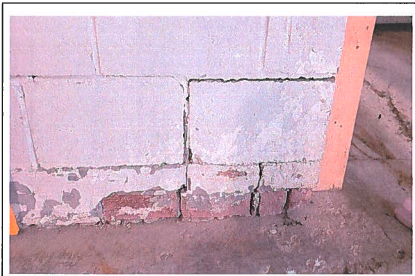
Photo 038 Block and Joint Damage
