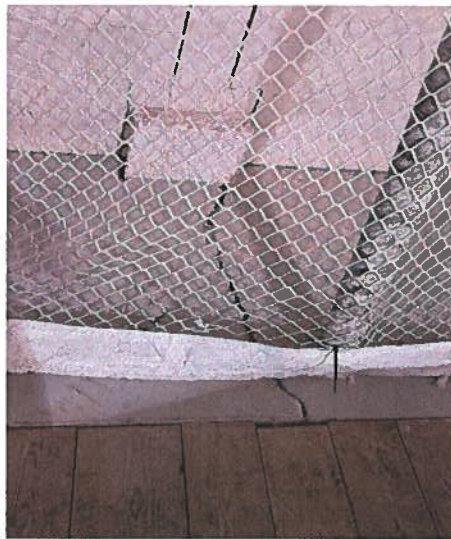
Photo 024 Cracking Under North-Side Column
