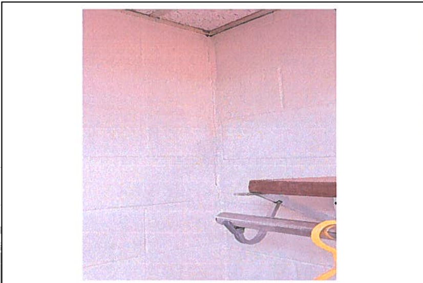
Photo 034 South-Side Stairwell Mortar Joint Cracking
