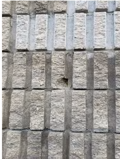
Photo 066 Localized Brick Damage
