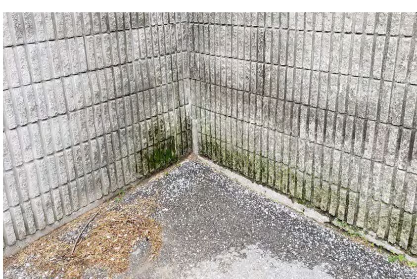
Photo 073 Moss Along East Side Wall
