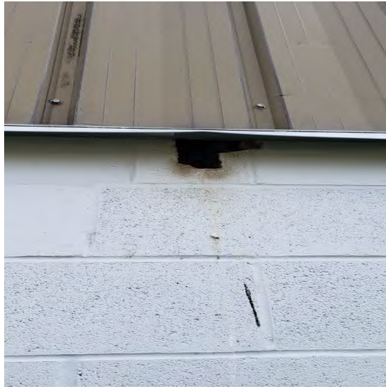
Photo 093 Hole in Masonry Block
