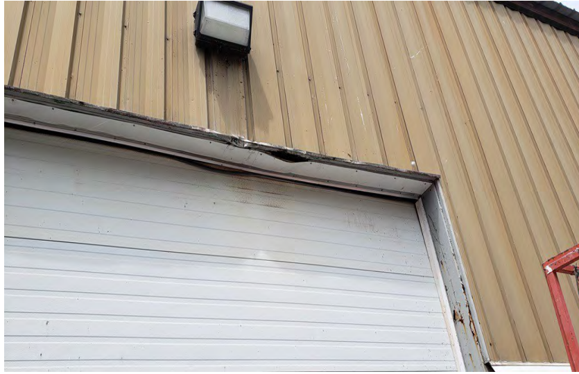
Photo 077 Damage to Garage Door Opening
