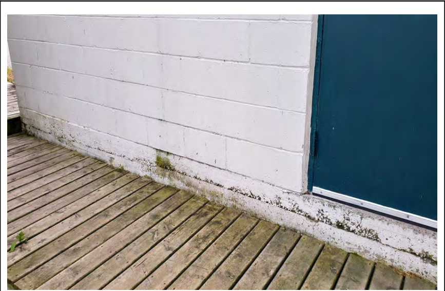
Photo 083 Honeycombing and Mould at Eastside of Ice-resurfacing Room
