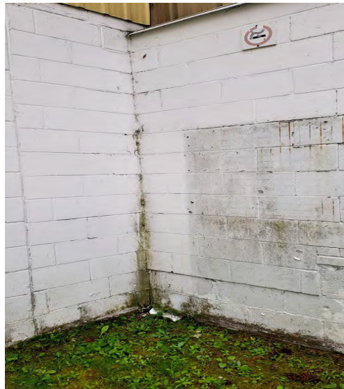
Photo 088 Mould and Moisture on Block Wal
