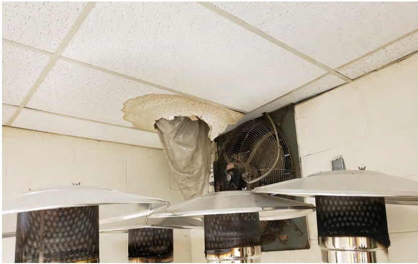
Photo 062 Signs of Moisture Damage
