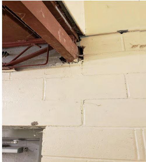
Photo 047 Localized Block Failure
