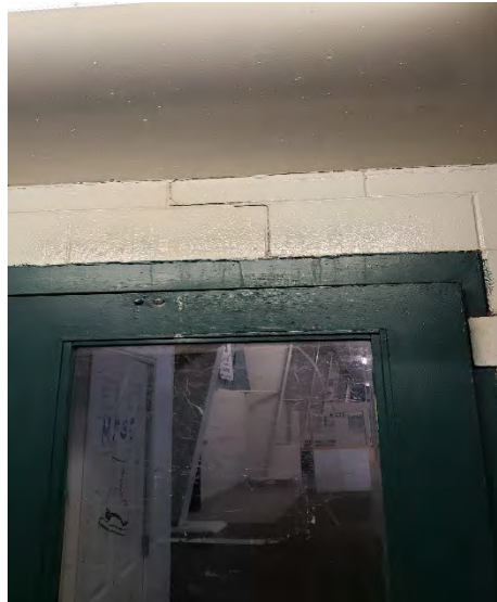
Photo 030 Step Cracking in Lobby
