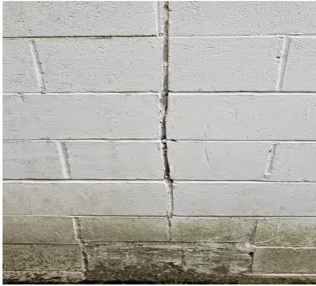
Photo 091 Damaged Wall Joint
