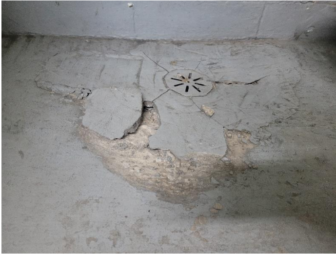
Photo 13 – Damaged Slab in Changeroom
