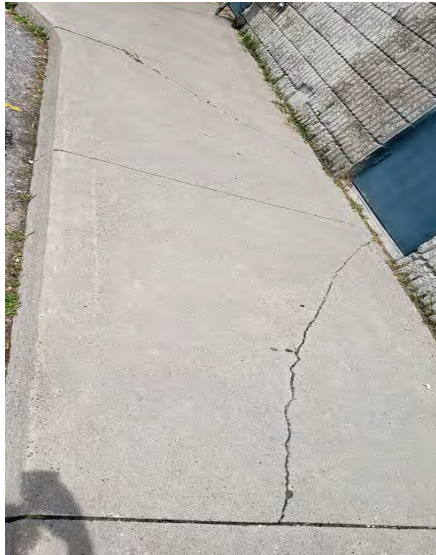
Photo 070 Damage to Sidewalk
