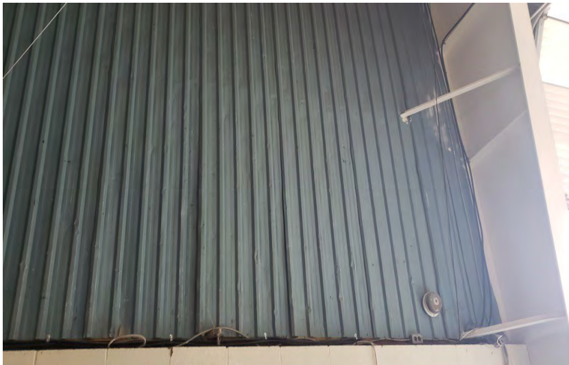
Photo 012 Localized damage to Metal Cladding
