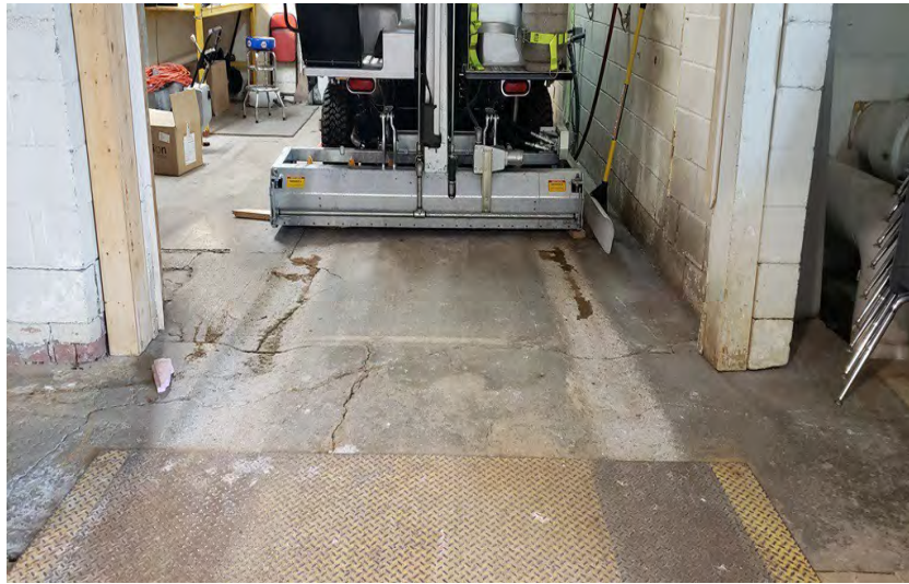
Photo 020 Resurfacing Room Rutting
