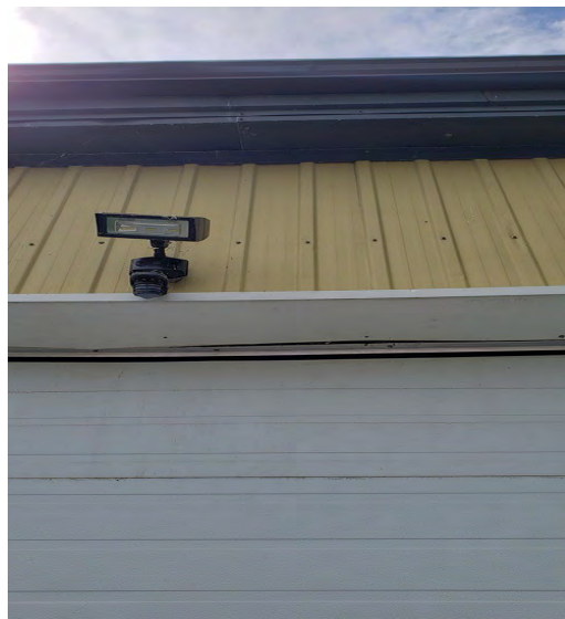
Photo 087 Damage to Garage Door Seal
