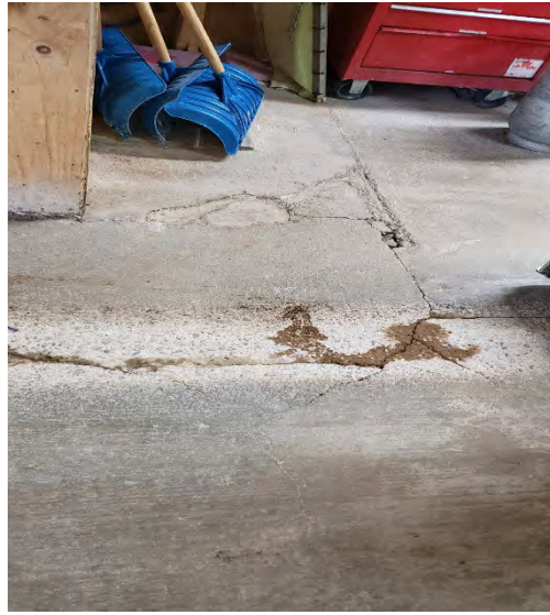
Photo 021 Cracking Starting in Resurfacing Room
