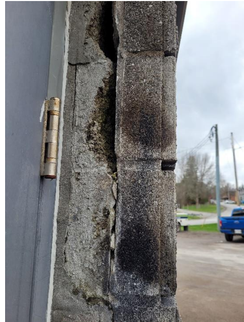
Photo 26 – Damaged Split Ribbed Block at Southwest Corner
