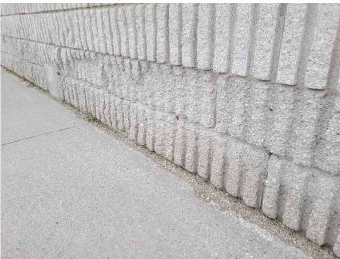
Photo 23 – Damaged Split Ribbed Block at Southeast Corner
