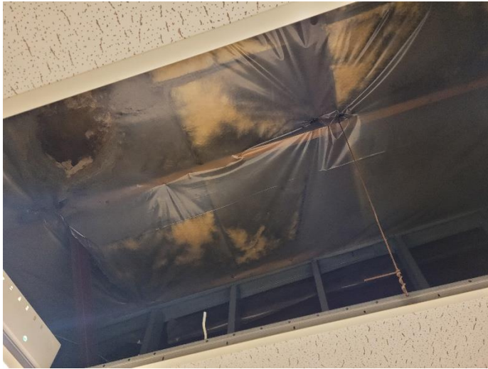
Photo 17 – Mould and Evidence of Moisture
