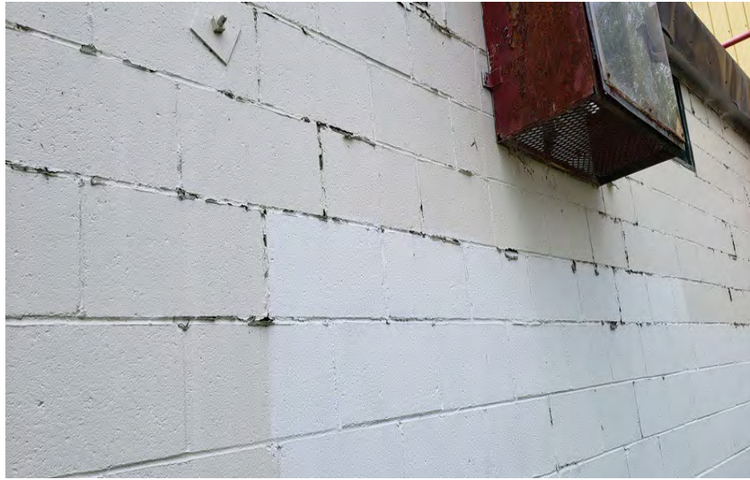
Photo 079 Step Cracking and Paint Peeling
