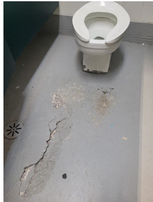
Photo 12 – Damaged Slab in Washroom
