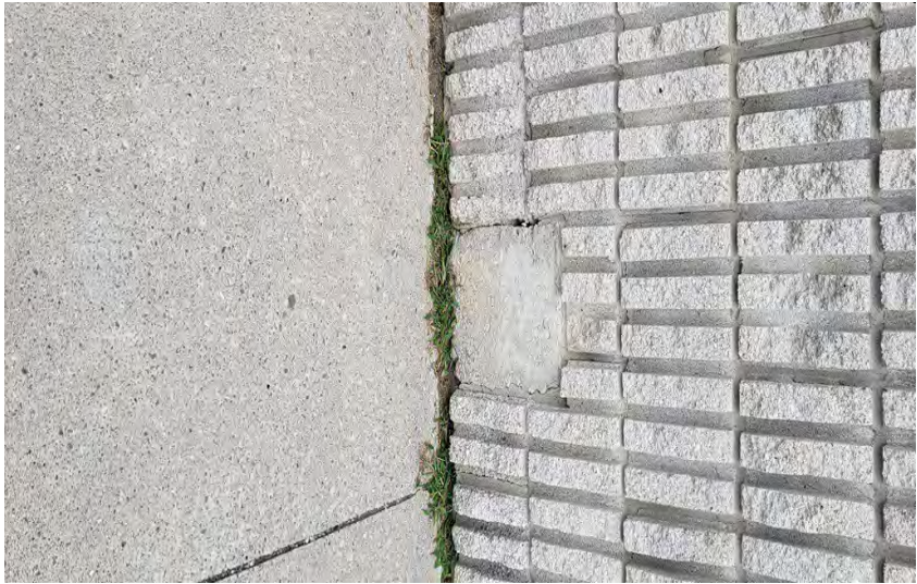
Photo 064 Cracking at Centre Foundation Wall
