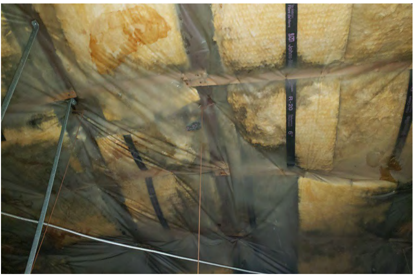
Photo 060 Moisture in Roofing System
