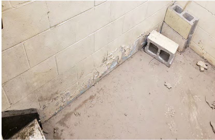
Photo 046 Paint Chipping and Moisture Damage
