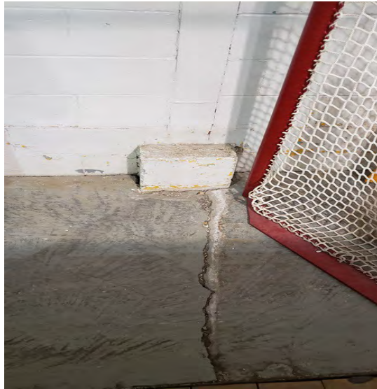
Photo 023 Cracking Under North-Side Column
