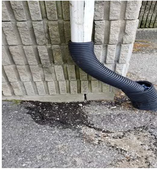
Photo 071 Gap in Foundation Wall
