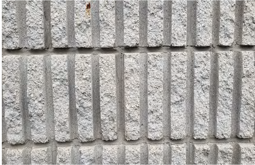
Photo 065 Architectural Block Mortar Cracks
