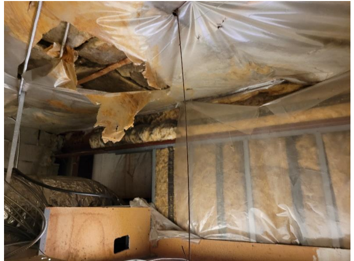
Photo 18 – Mould and Evidence of Moisture
