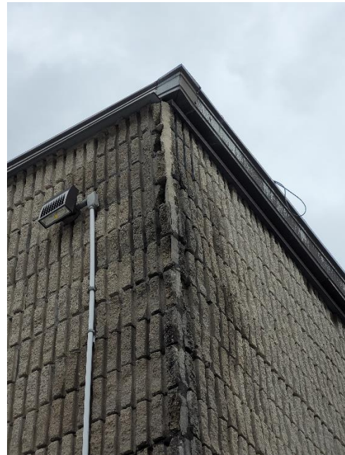
Photo 22 – Damaged Split Ribbed Block at Southeast Corner
