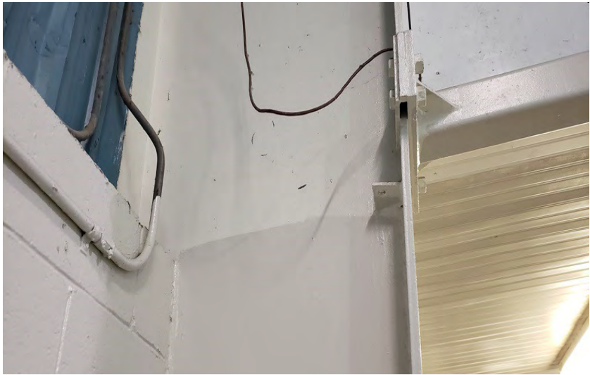
Photo 008 Missing Brace at Southmost Frame
