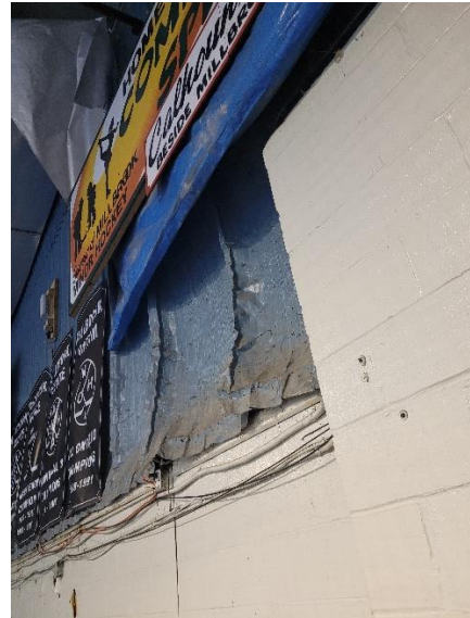
Photo 02 – Damaged Metal Siding
