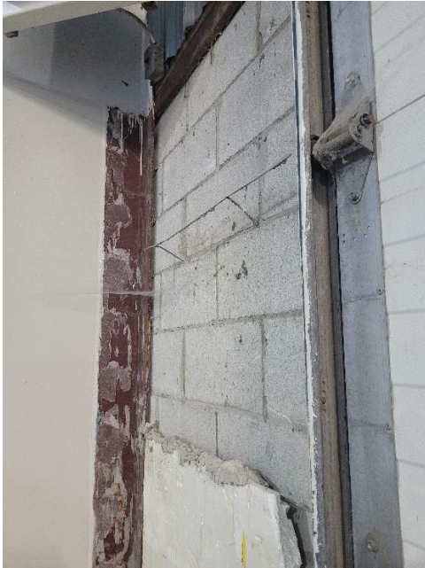
Photo 05 – Damaged Block Wall
