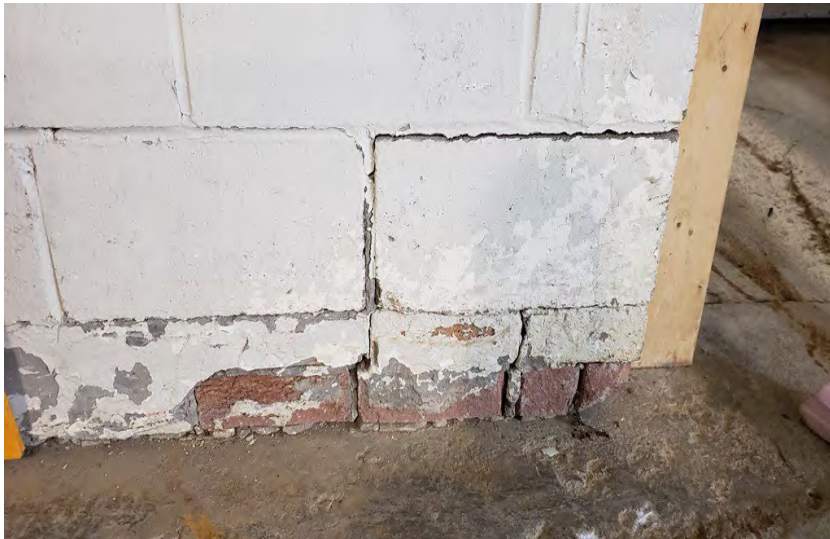
Photo 038 Block and Joint Damage
