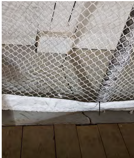
Photo 024 Cracking Under North-Side Column
