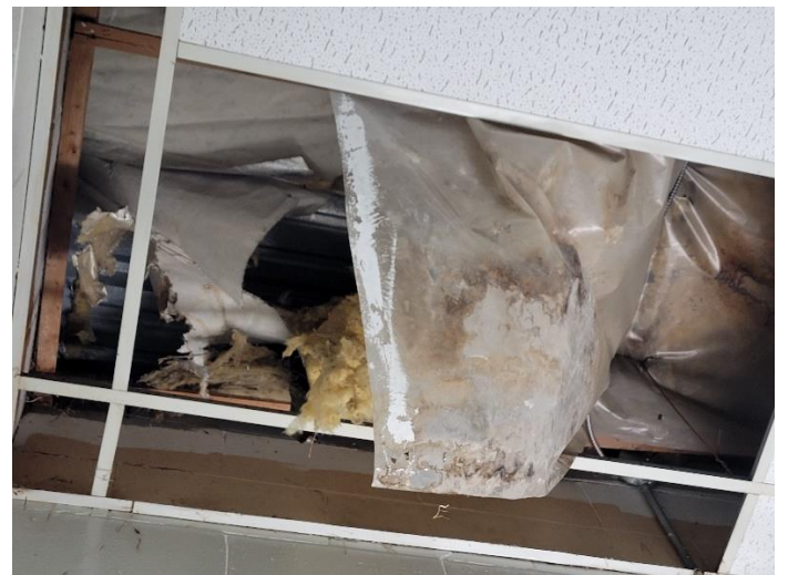
Photo 16 – Damaged Roof Insulation and Evidence of Moisture
