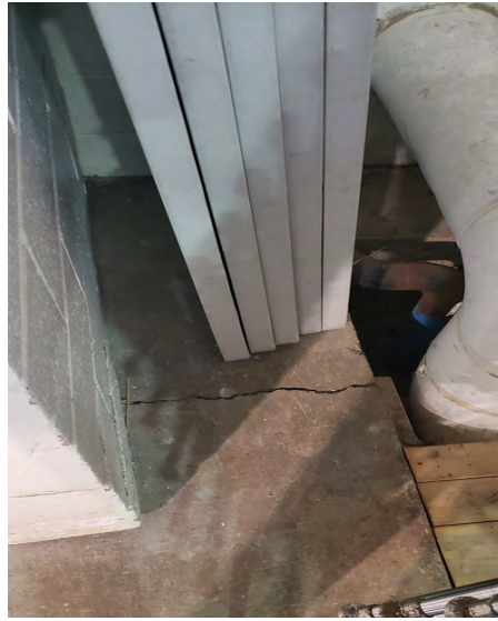
Photo 019 Major Crack in Apron Slab
