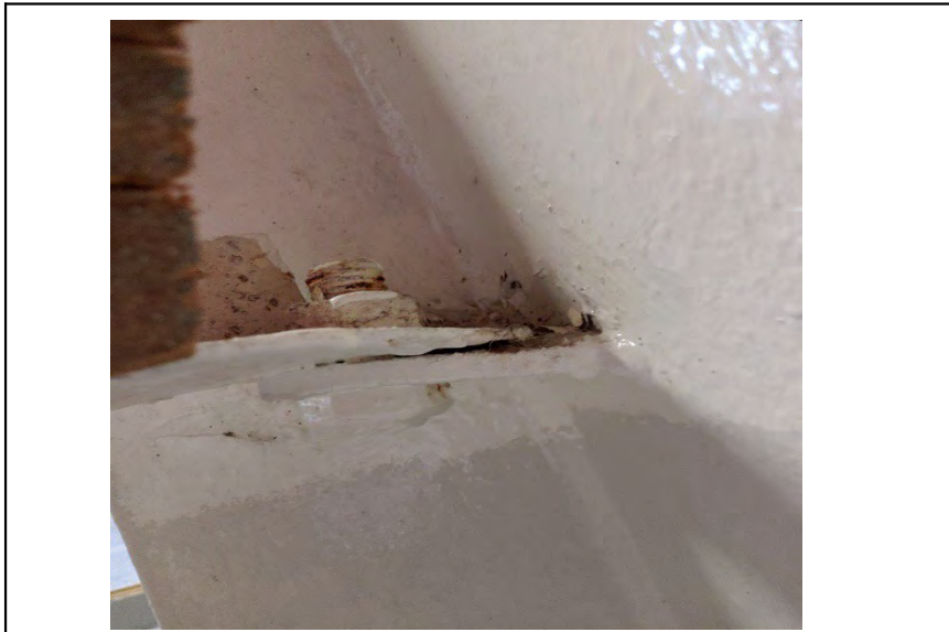
Photo 006 Rusted Bracing Connection
