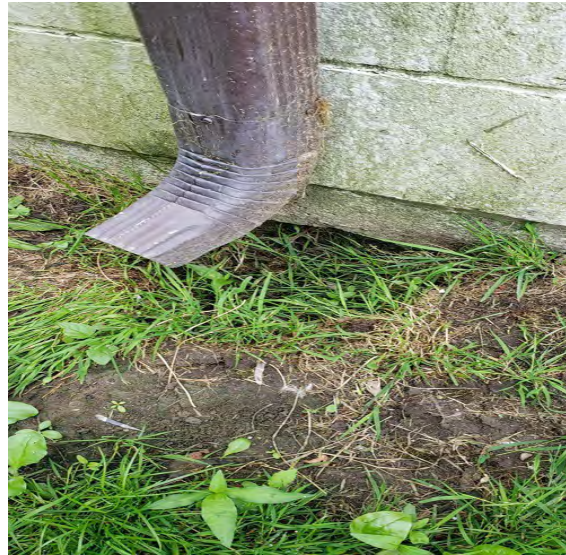
Photo 092 Localized Foundation Wall Damage
