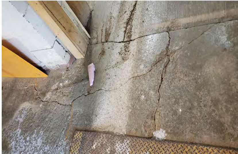
Photo 022 Extents of Resurfacing Room Cracking
