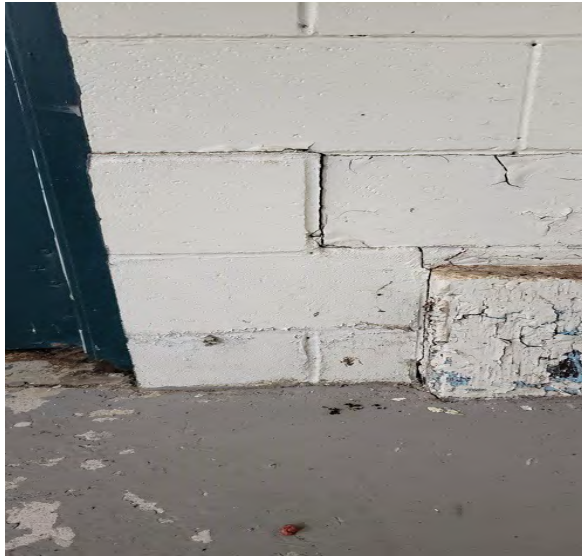
Photo 039 Step Cracking and Damage to West-Side Exit
