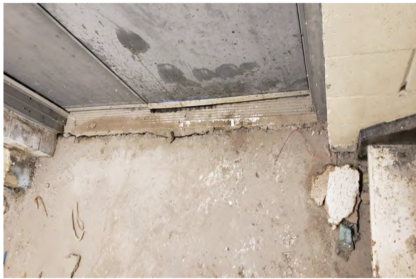
Photo 054 Slab-On-Grade Damage in West-Side Stairwell
