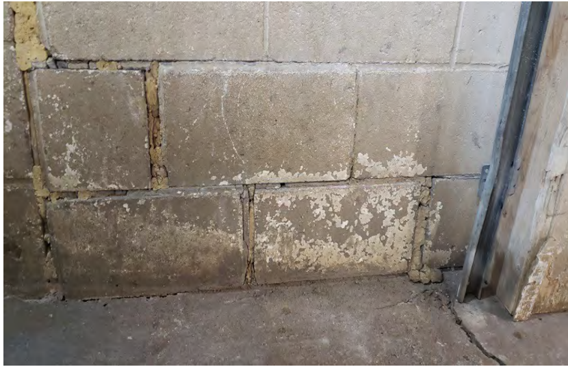
Photo 037 Existing Block Separation Repairs
