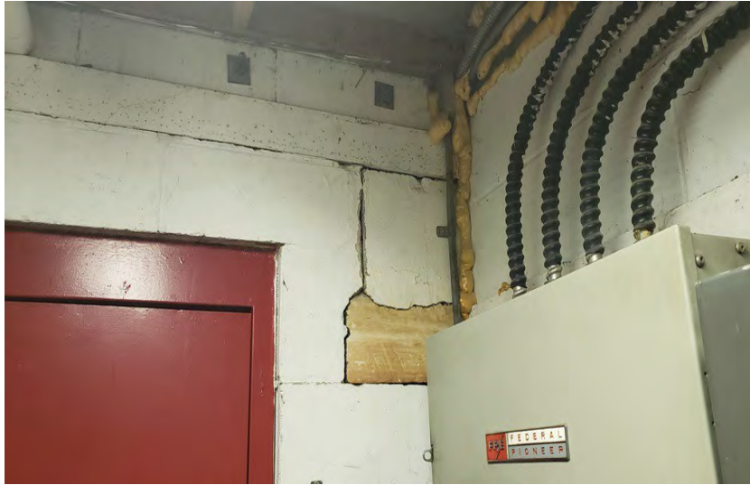
Photo 035 Wooden Block Replacement and Cracking
