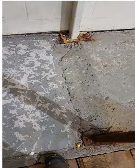
Photo 025 Crack Underneath Mechanical Equipment Stand
