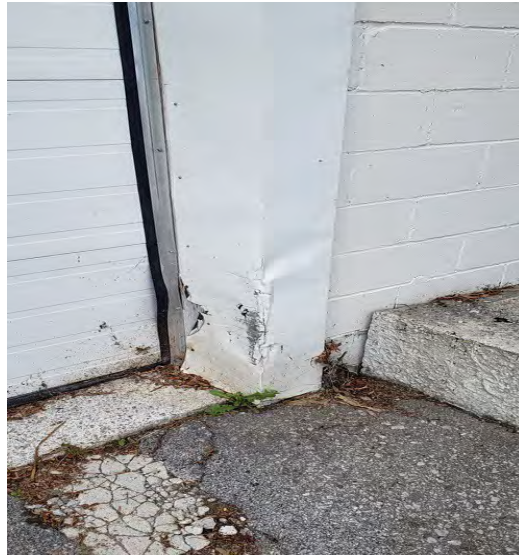
Photo 086 Damage to Garage Door Entrance
