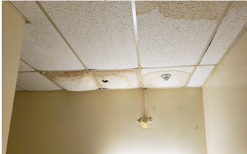
Photo 061 Signs of Moisture Damage
