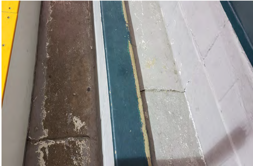
Photo 011 Bleacher Crack at Joint Location
