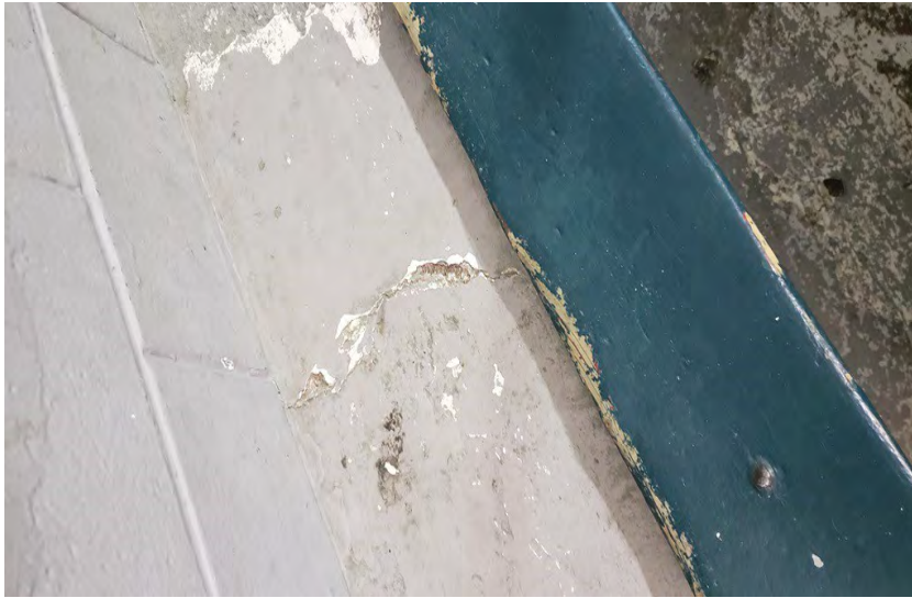
Photo 010 Paint Chipping and Crack on Bleachers
