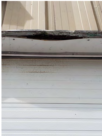
Photo 078 Close Up of Damage Garage Door
