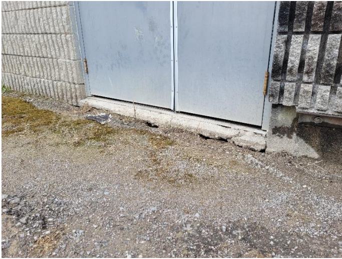
Photo 25 – Damaged Concrete Slab at Southwest Corner
