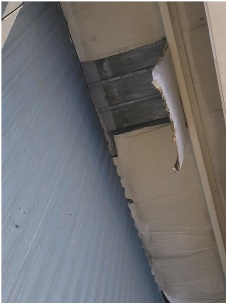
Photo 03 – Damaged Roof Insulation
