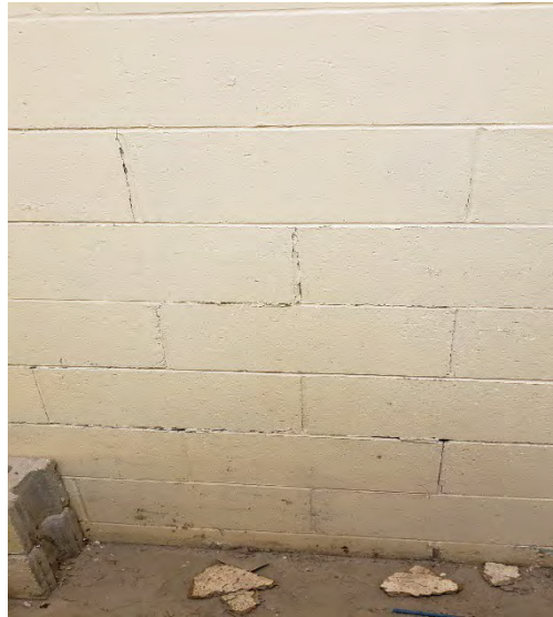
Photo 031 Minor Step Cracking in West-Side Stairwell
