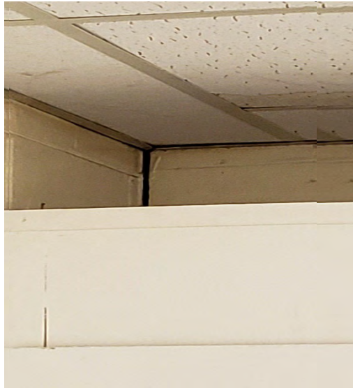
Photo 049 Wall Separation in Second-Floor Storage Room
