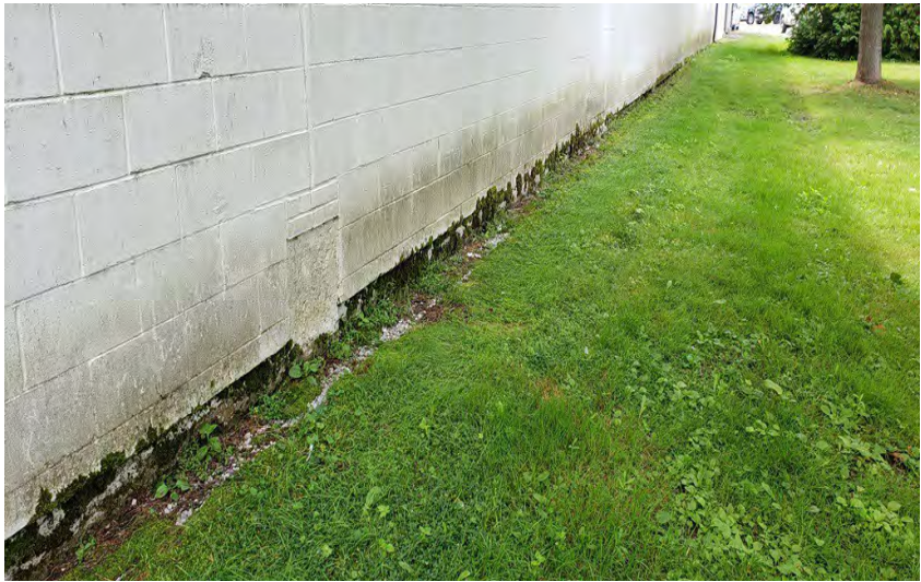
Photo 090 Mould Along West Side
