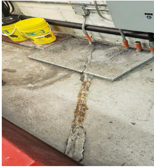
Photo 053 Concrete Damage at Electrical Equipment in Compressor Room
