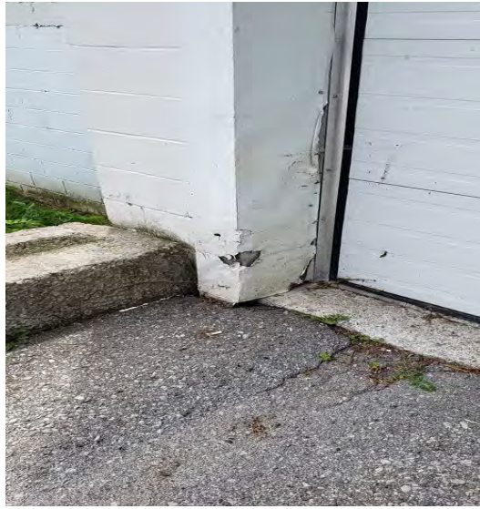
Photo 085 Damage to Garage Door Entrance
