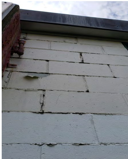
Photo 080 Step Cracking and Paint Peeling
