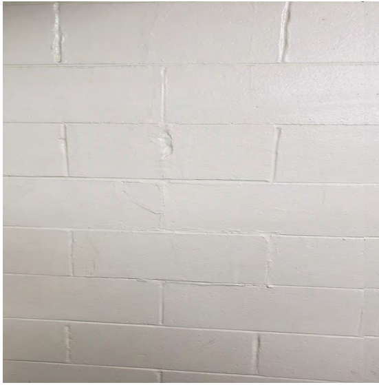
Photo 043 Localized Damage in Changeroom 3
