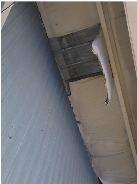
Photo 03 – Damaged Roof Insulation
