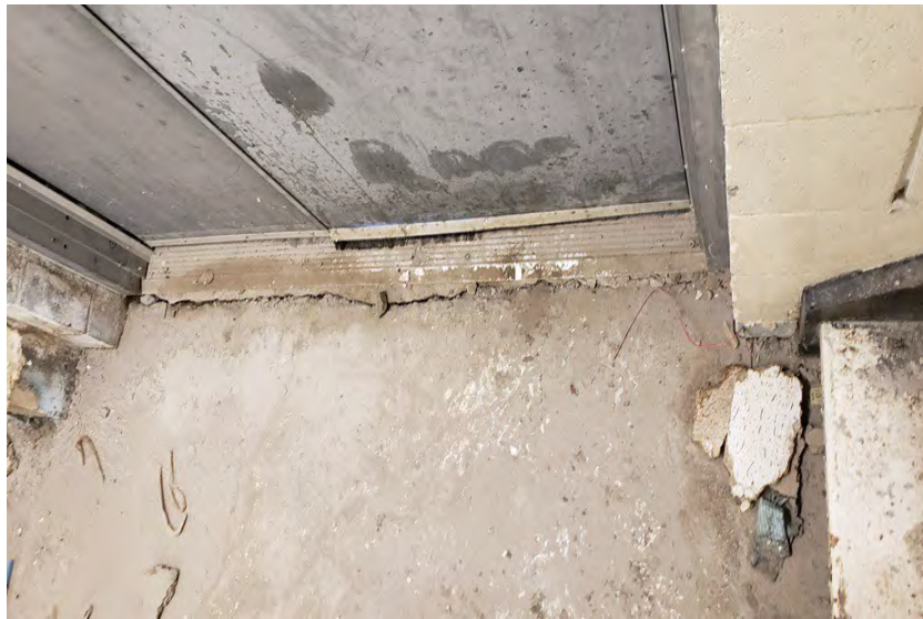
Photo 054 Slab-On-Grade Damage in West-Side Stairwell
