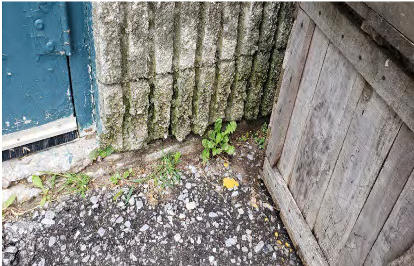
Photo 074 Deterioration of Blocks
