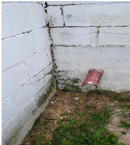
Photo 082 Honeycombing and Mould Growth
