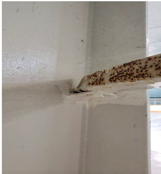
Photo 004 Rust on Frame Brace
