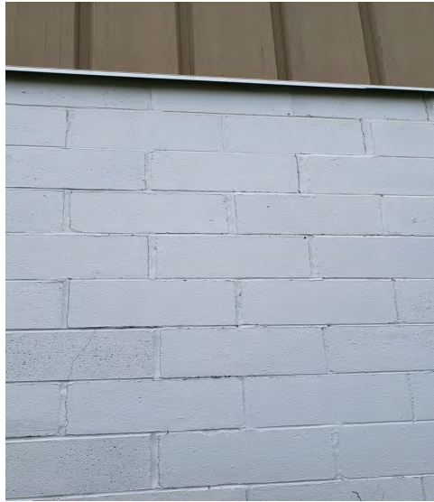
Photo 081 Step Cracking and Block Failure
