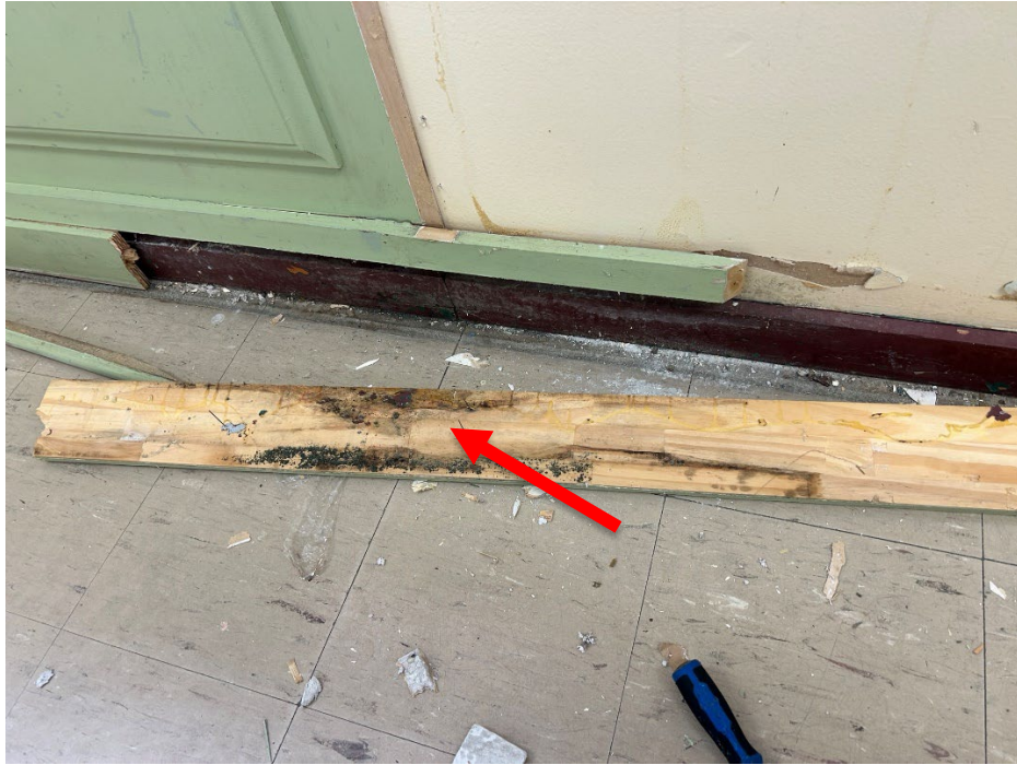
Photo 13 Mould impacted wooden baseboard.
