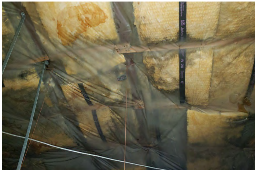
Photo 060 Moisture in Roofing System
