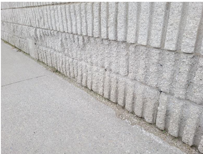
Photo 23 – Damaged Split Ribbed Block at Southeast Corner
