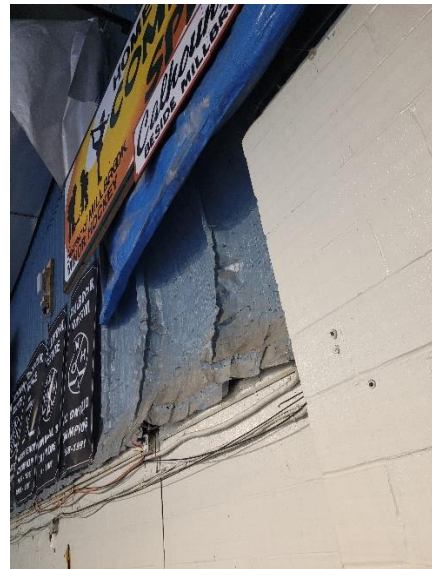
Photo 02 – Damaged Metal Siding
