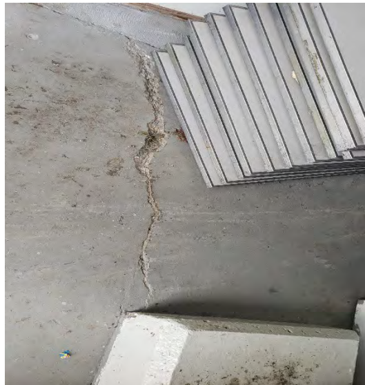
Photo 017 Cracking Outside of Compressor Room
