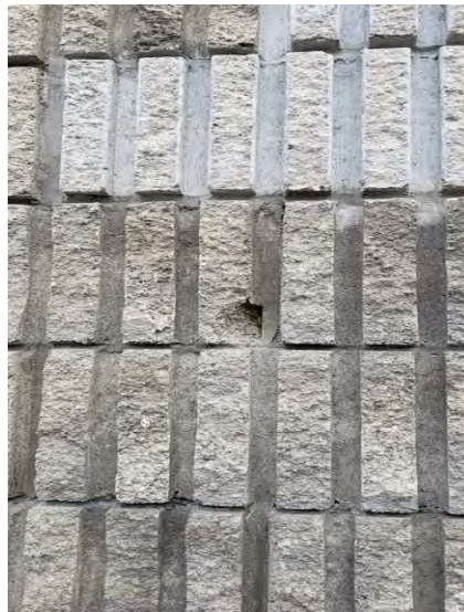
Photo 066 Localized Brick Damage
