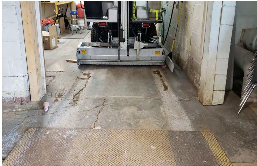
Photo 020 Resurfacing Room Rutting
