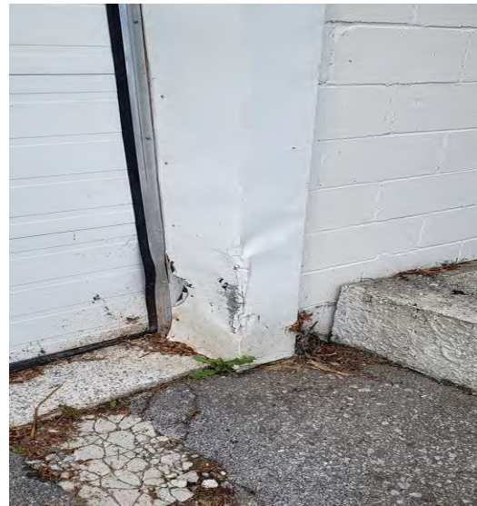
Photo 086 Damage to Garage Door Entrance
