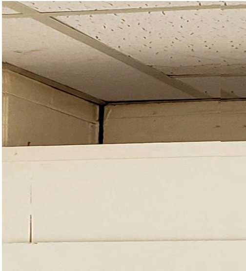
Photo 049 Wall Separation in Second-Floor Storage Room
